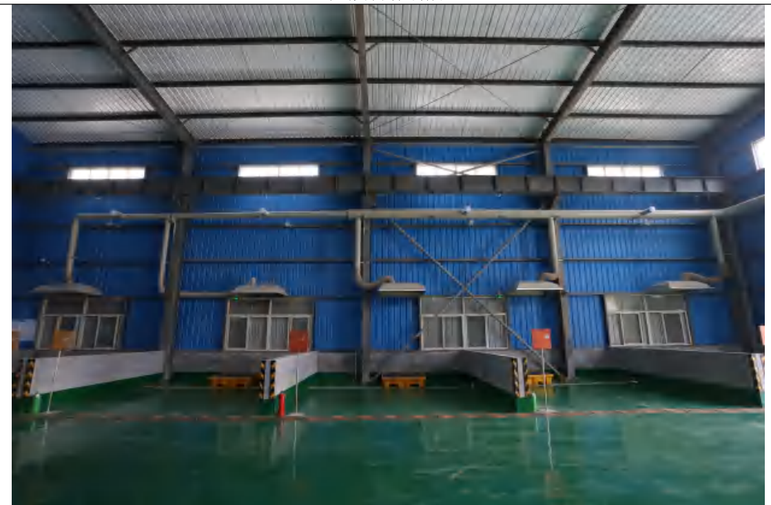
危废暂存分区且设置集气罩
