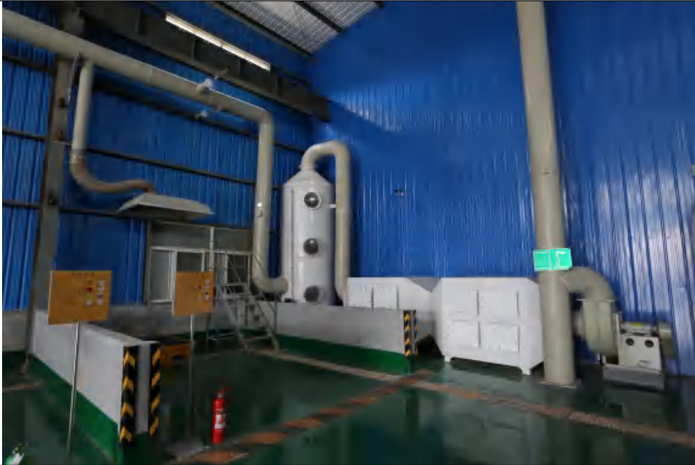
碱喷淋+二级活性炭装置+15m 排气筒
